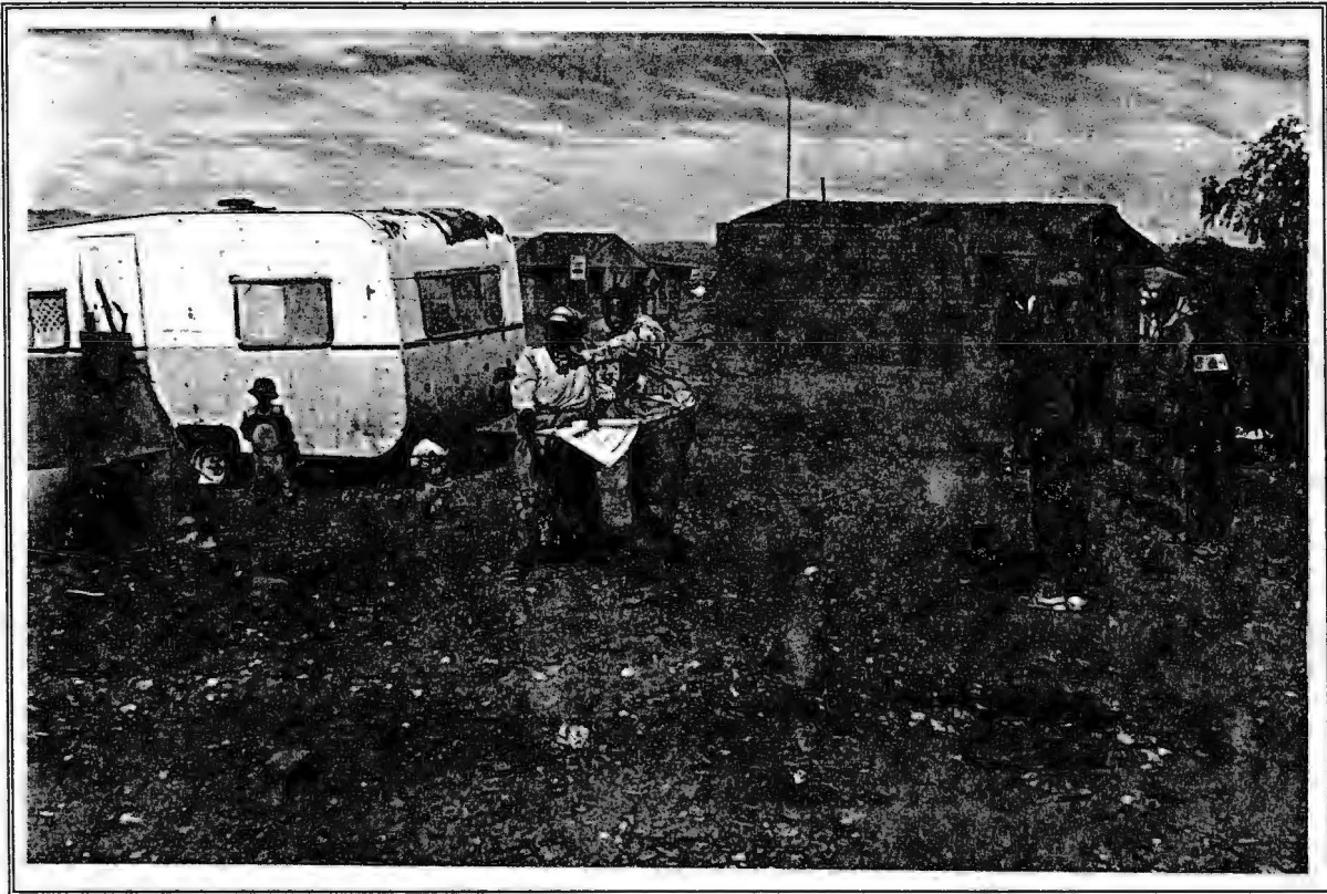
Mr. Attie Swartz, one of the Programme's self-help construction advisors explains to a client the possible location of her house. In the background, another starter solution under construction can be seen.
