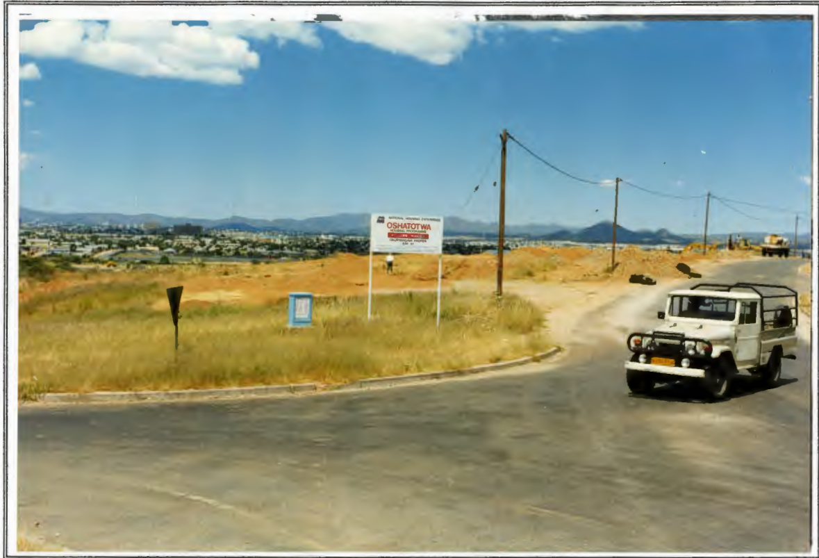
Infrastructure works are well underway on two Core-House project sites, in Khomasdal and Okuryangava. Trenches for water, electricity and sewage are already dug on this site in Okuryangava.
