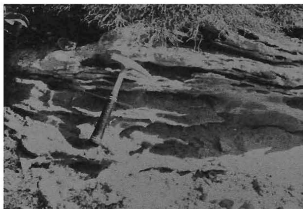
Figure 25 Thick and very thick platy hardpan calcretites with intervening sand lenses exposed in road cutting at Saldanha Bay, Cape Province.
