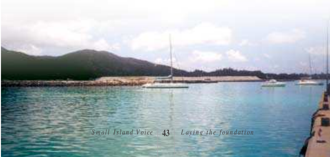
Land reclamation, as seen here at Baie Ste Anne, Praslin, Seychelles, provides flat land for housing and other development, 2002.
