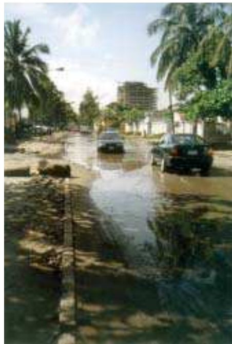
Blocked drainage channels result in frequent flooding during the rainy season, Lagos, Nigeria, July 2002.
