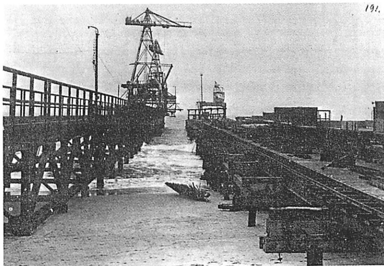
On the right the old wooden jetty, on the left the iron jetty under construction.
