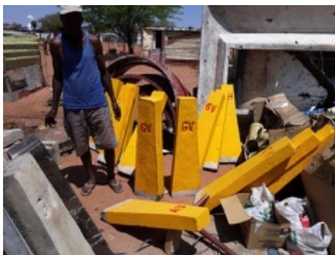
Construction of concrete signs for gate valves and fire hydrants is also done by SDFN/NHAG
